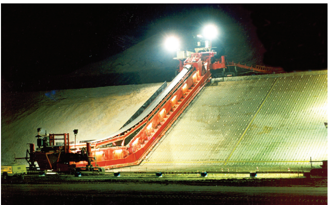
Night lighting system illuminates not only the G&Z Canal Liner but much of the surrounding area.
